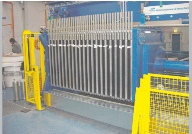
Filter press with membrane- and combination chamber plates 1200 x 1200 mm. Filtration of metal pigments with solvents, 16 bar squeezing pressure
